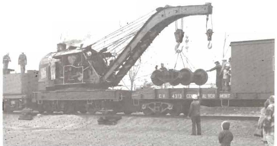
The Society's ex-Central Vermont steam crane 4251 at work in the late 1970s. (BRS Collection)
