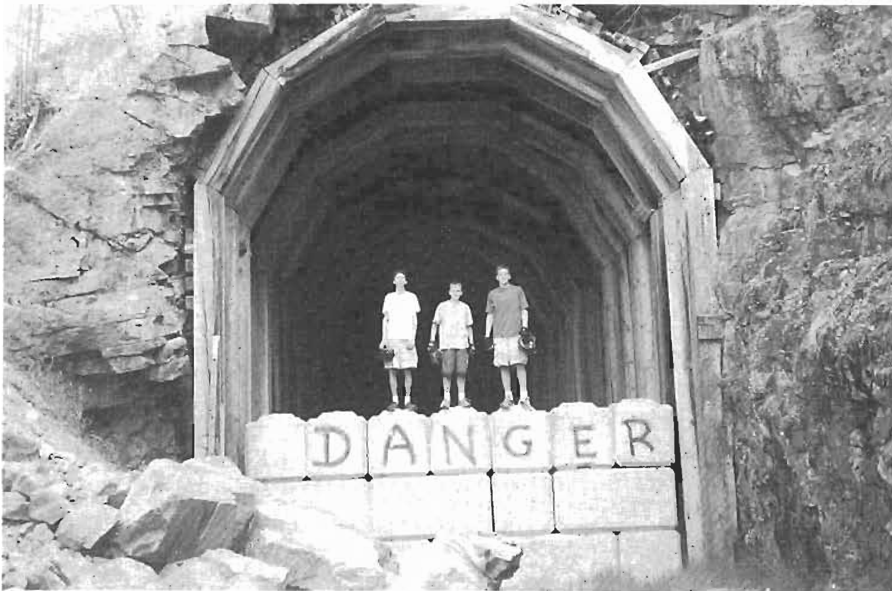
The south portal of the Adra Tunnel, closed to cyclists since 1992 because of falling debris.
