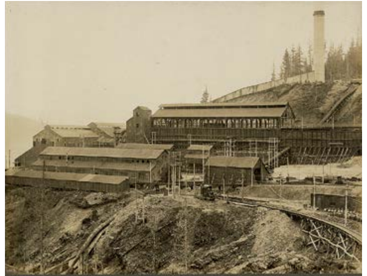
1. Smelter under construction, showing rail trackage used to assist in the construction. In the foreground to the left of the trestle is a steam-powered rail-mounted crane. Photograph reproduced by permission of UBC Archives (Accession Number BC1456-7-42).
