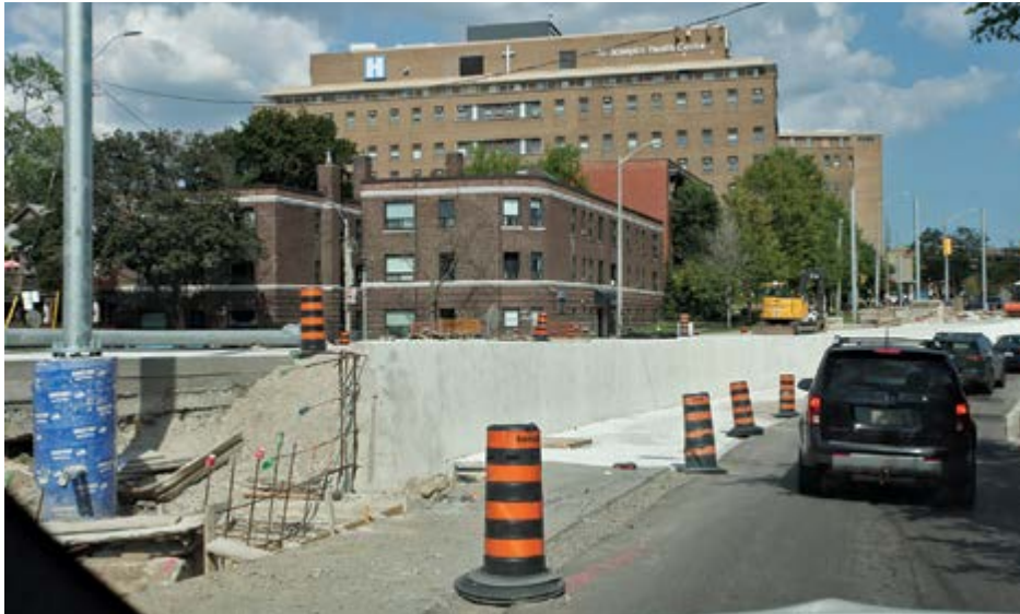
Above - This is a view about 200 metres west of Roncesvalles Junction in the middle of construction.
