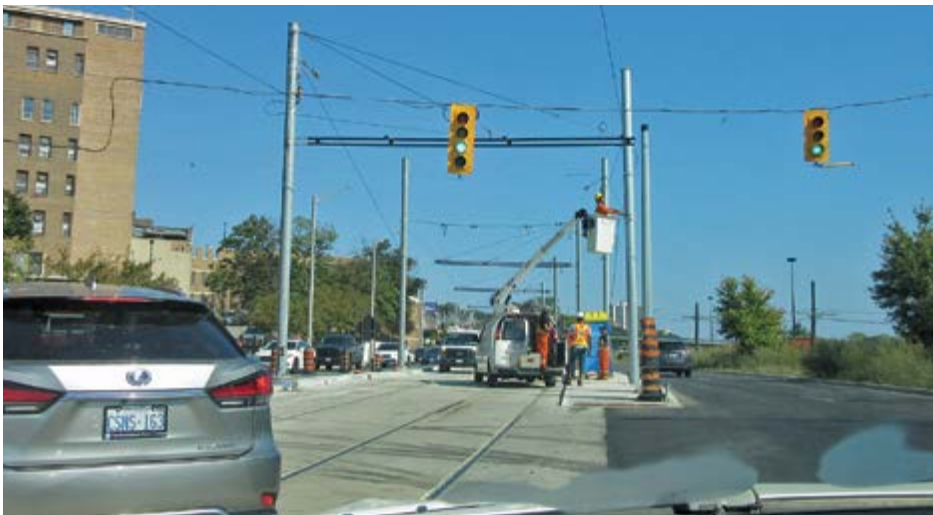
Below - This is a second photo taken on Wednesday September 6. All that is missing is a few hundred feet of overhead wire at this location. Workers can be seen doing electrical work. By the time you get your next copy of Branchline the line should be open. Both photos by Gerald Harper
